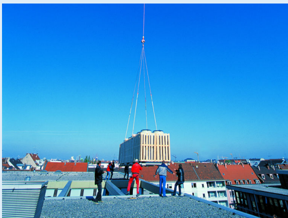
Güntner's V-coil drycoolers are placed by helicopter exactly where they are needed, on the roof of the Ludwig Maximilian University opposite the Alte Pinakothek.
