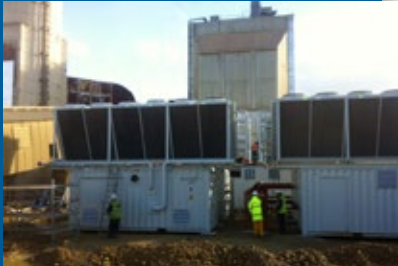
▲ Four Güntner air-cooled V-SHAPE Vario GVD condensers are part of the Heatcatcher ORC system generating electricity from waste heat for own requirements.
